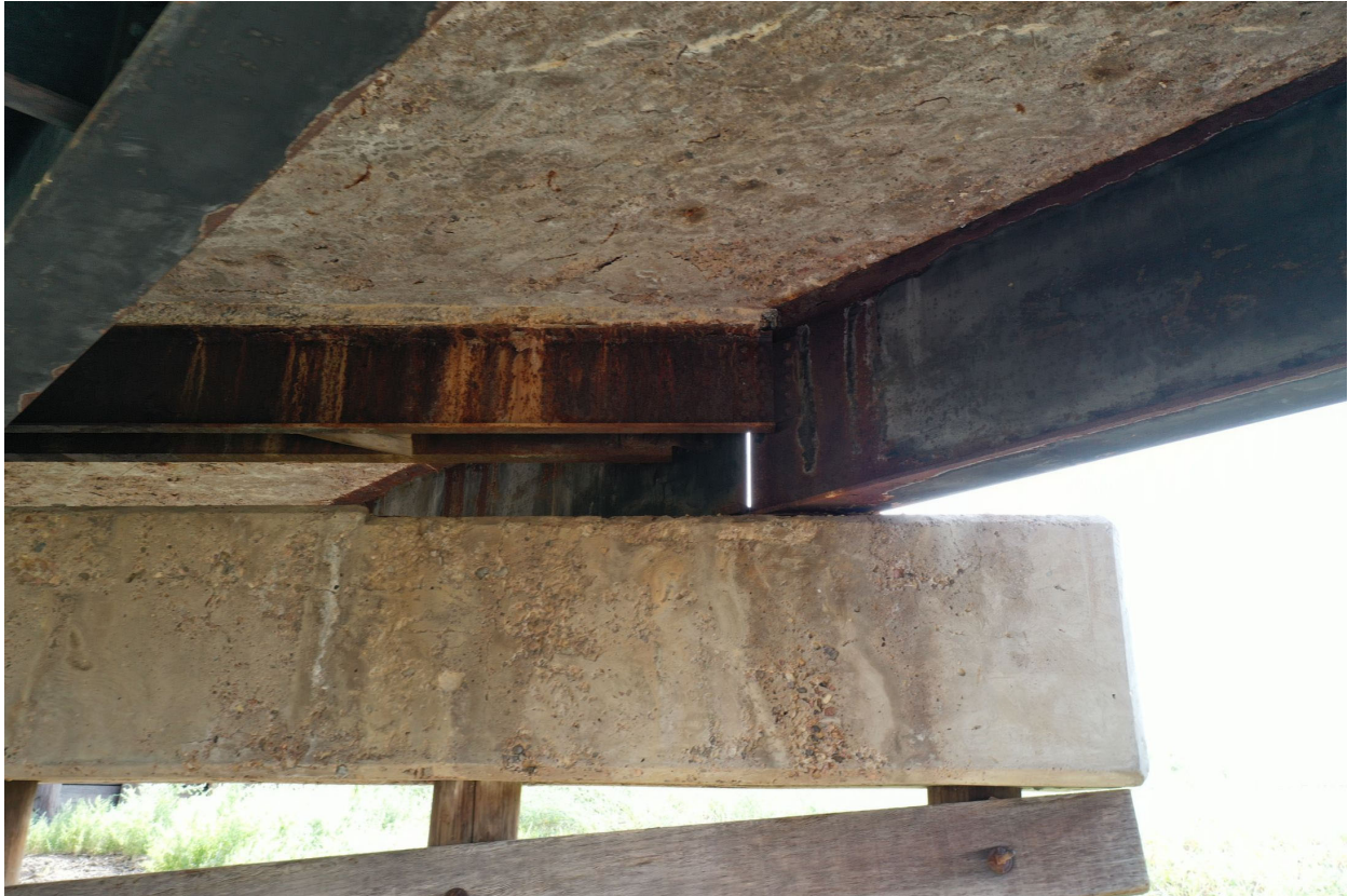
Picture 3 - Corrosion, Exposed Aggregate
